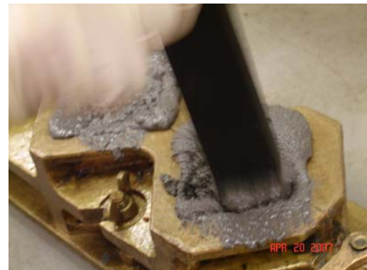
Fill molds halfway with epoxy grout then tamp or rod to remove entrapped air.
