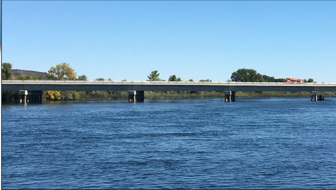
Badly Damaged Piles Prior to Repair
