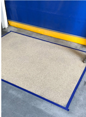
Broadcast calcined Bauxite applied over epoxy coating and RSR Easy Mix™ resulting in an R14 non-slip surface.
