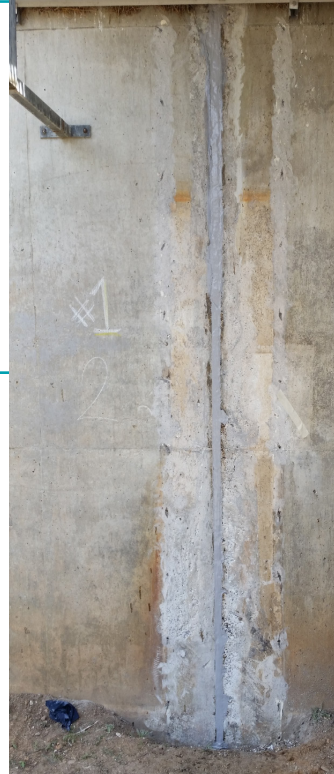
Five Star Structural Concrete® V/O applied to repair vertical expansion joint in clarifier.
